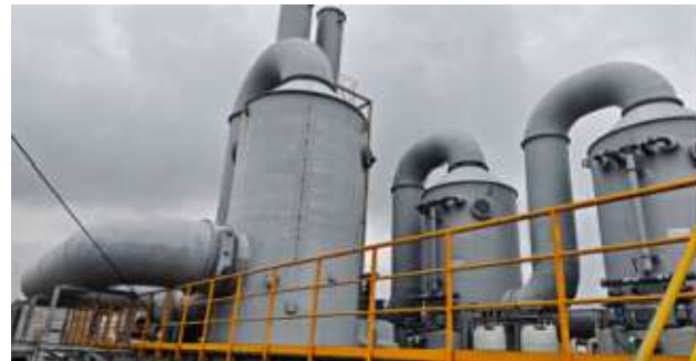
Waste gas treatment facilities
