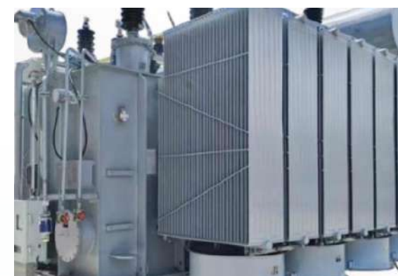
630KVA transformer capacity
