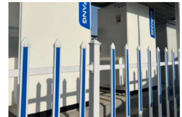
522kWh energy storage station
