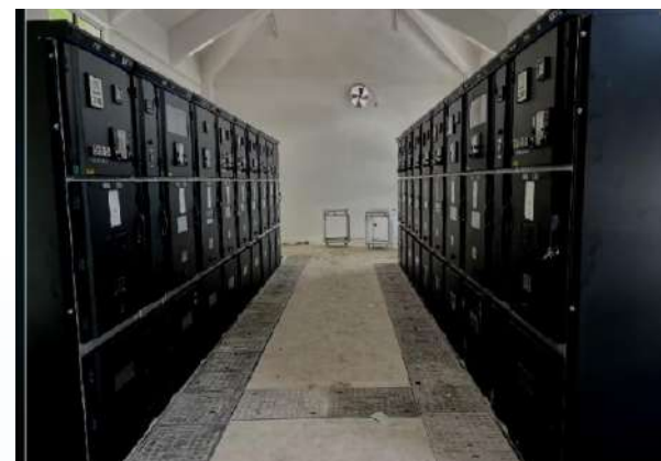
Intelligent distribution room of Hubei University
