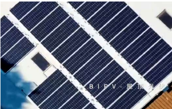
BIPV Roof Photovoltaic Panel
