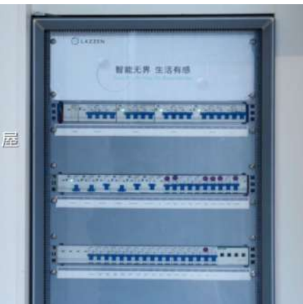
Whole-House Intelligent Control System
