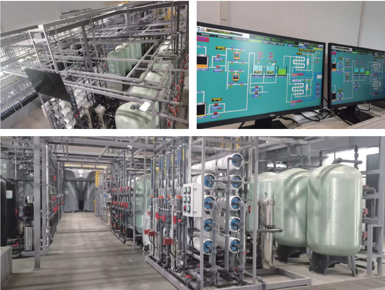
LAZZEN's electroplating wastewater treatment system
